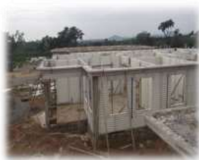
Plate 6: EPS Fascia (Cornices) are carefully strongly tied to the walls using wires and splice meshes
