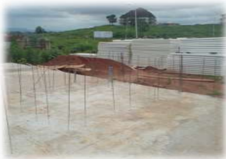
Plate 2: Starter Bars of Diameter 10mm are inserted At 500mm c/c before oversite concrete is cast
