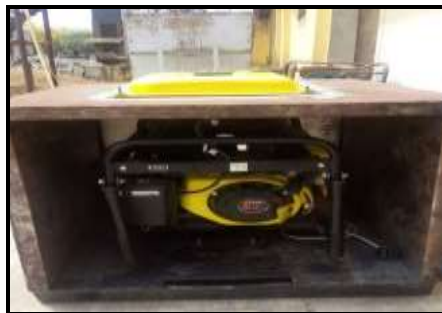
Figure 3: Enclosure and 2KVA Electric Power Generator
