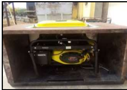
Figure 3: Enclosure and 2KVA Electric Power Generator
